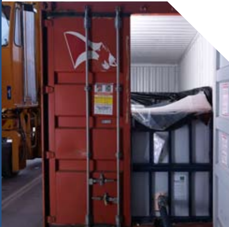
Grundfos Hilge SIPLA pumps extract wine from shipping containers, bringing it into Accolade's processing plant.
