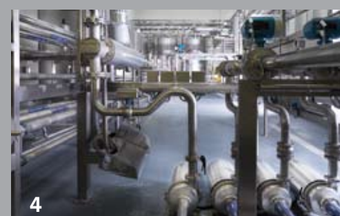
Left: Grundfos Hydro booster set for main water supply. Above: hot water circulation pumps (1); distribution centre (2); high-speed bottling line (3); Clean In Place pumps for cleaning interiors of pipes and process equipment (4).
